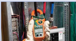
Collecting current measurements and associating them with the right component identified on an infrared image, can be a complicated and cumbersome process
